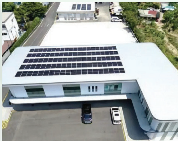
Sikarin Solar Rooftop Project (Ongrid)
